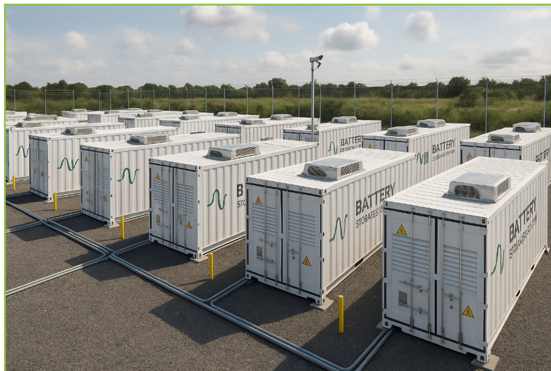
Figure 7 Grid Scale Deployment
